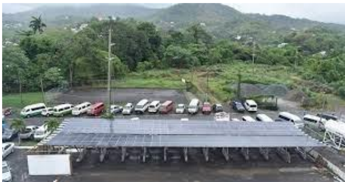
Figure 15: Solar carport facility at the Ministry of Infrastructure, Ports and Energy (Union, Castries) in Saint Lucia.
