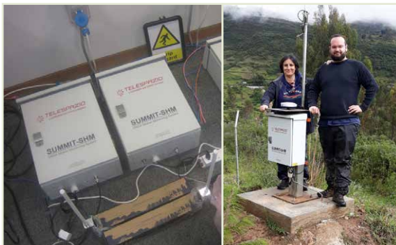
Installation of SUMMIT-SHM equipment at Colquirrum
